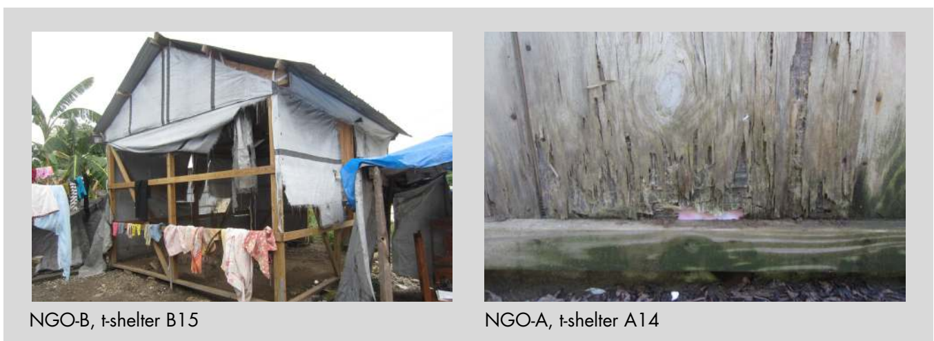
Figure 1: Examples of eroding t-shelters
