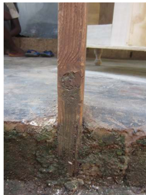
Figure 18: Slowly the elements deteriorate t-shelters (t-shelter A8)
