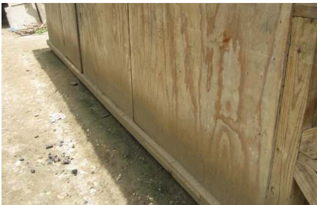
Figure 17: Rain-damaged plywood (t-shelter A29)
