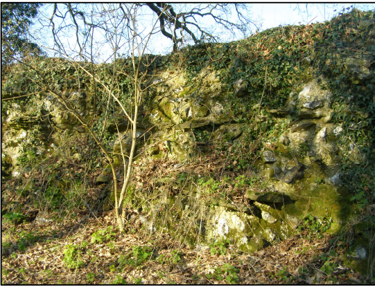
Figure 4.4: Un-restored section. Hedera helix (ivy) and trees can be seen covering the wall (Source: author).
