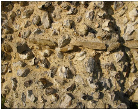
Figure 4.1: Section of the south wall, restored with Portland cement. Note Portland cement's characteristic white colour, and see that large areas are covered with the cement (Source: author).
