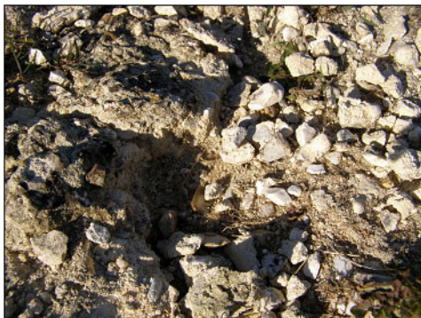
Figure 4.2: Section of the north-east facing wall, restored with lime mortar. Note its decomposition and 'crumbly' appearance, the whole area looked like this (Source: author).
