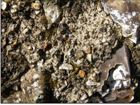
Figure 4.3: Section of the north-east facing wall, restored with cement mortar. This material was also hard, and did not crumble as the lime mortar (Source: author).
